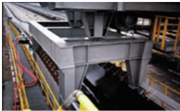
Figure 3. Head of conveyor at transfer tower
