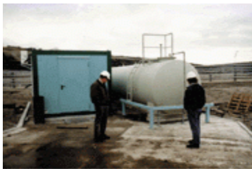
Figure 1. Dust suppression system and chemical storage tank at Schleenhain mine
