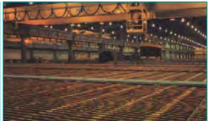
“Electrowinning” - is electroplating of dissolved copper onto metal anodes using electrical current
